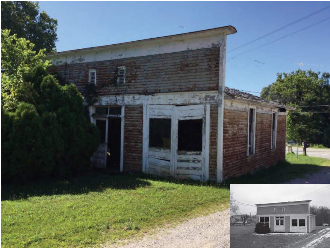
Photo ID 790, August Meyer House and Meyer Undertaker Shop, potentially NRHP-eligible, 2572 E SR 56, Dubois Co.; Alternative O
