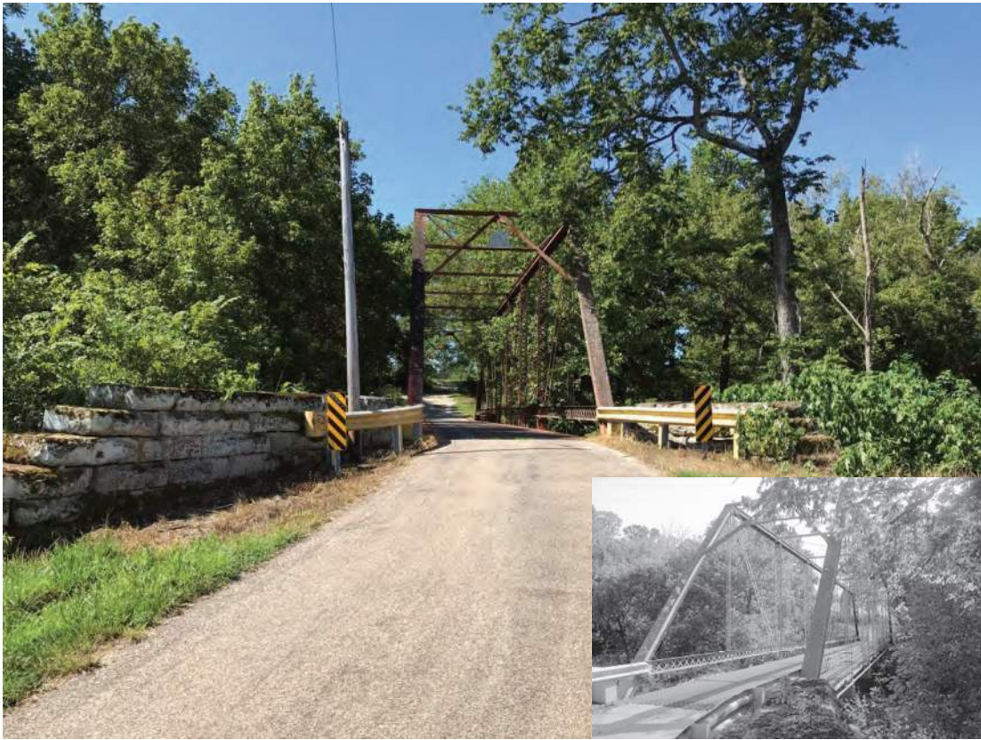
Photo ID 1064, Orange Co. Bridge No. 31, potentially NRHP-eligible, CR 525 W over Lost River, Orleans; Alternative O
