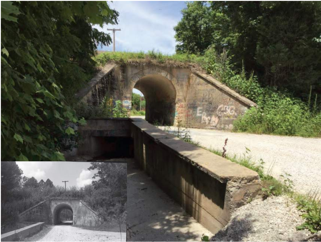
Photo ID 866, Railroad Bridge, potentially NRHP-eligible, S. Hillham Road, Orange Co.; Alternative O
