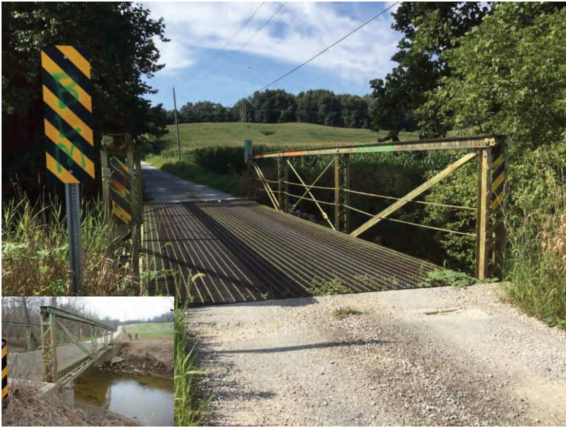
Photo ID 1235, Martin Co. Bridge No. 67, potentially NRHP-eligible, CR 33 over Friends Creek; Alternatives M, P
