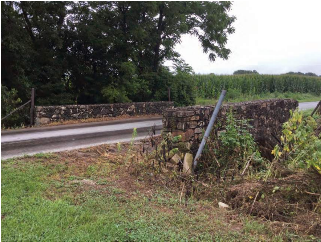
Photo ID 1097, Bridge, potentially NRHP-eligible, CR 200 W over Mount Horeb Drain, Lawrence Co.; Alternative O
