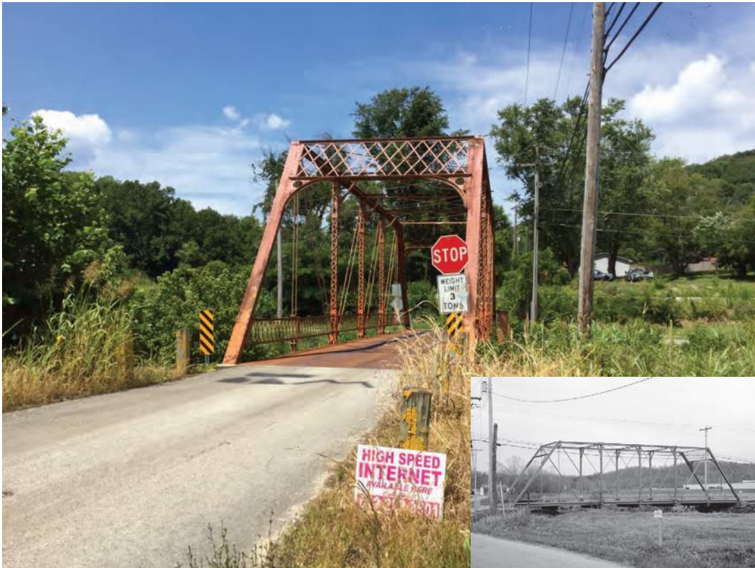
Photo ID 854, Orange Co. Bridge No. 49, potentially NRHP-eligible, CR 100 S over French Lick Creek, French Lick; Alternative O
