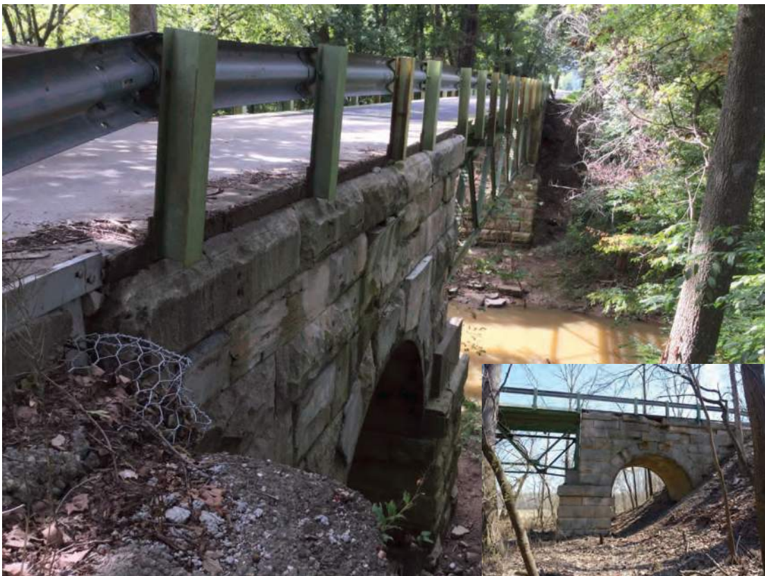
Photo ID 1283, Martin Co. Bridge No. 58, potentially NRHP-eligible, Brickyard Road over Boggs Creek; Alternatives M, P
