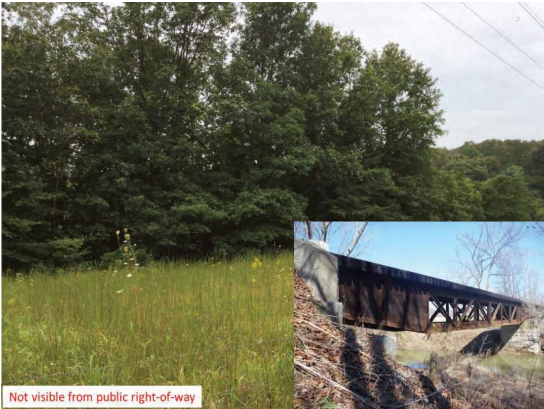
Photo ID 1608, Railroad Bridge, potentially NRHP-eligible, between Cale Road and Low Gap Road, Martin Co.; Alternative M
