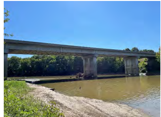
Figure 16. West side of US 231 bridge from north bank of East Fork White River
